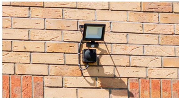
Rear security light with PIR
