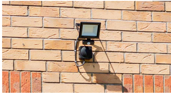
Rear security light with PIR
